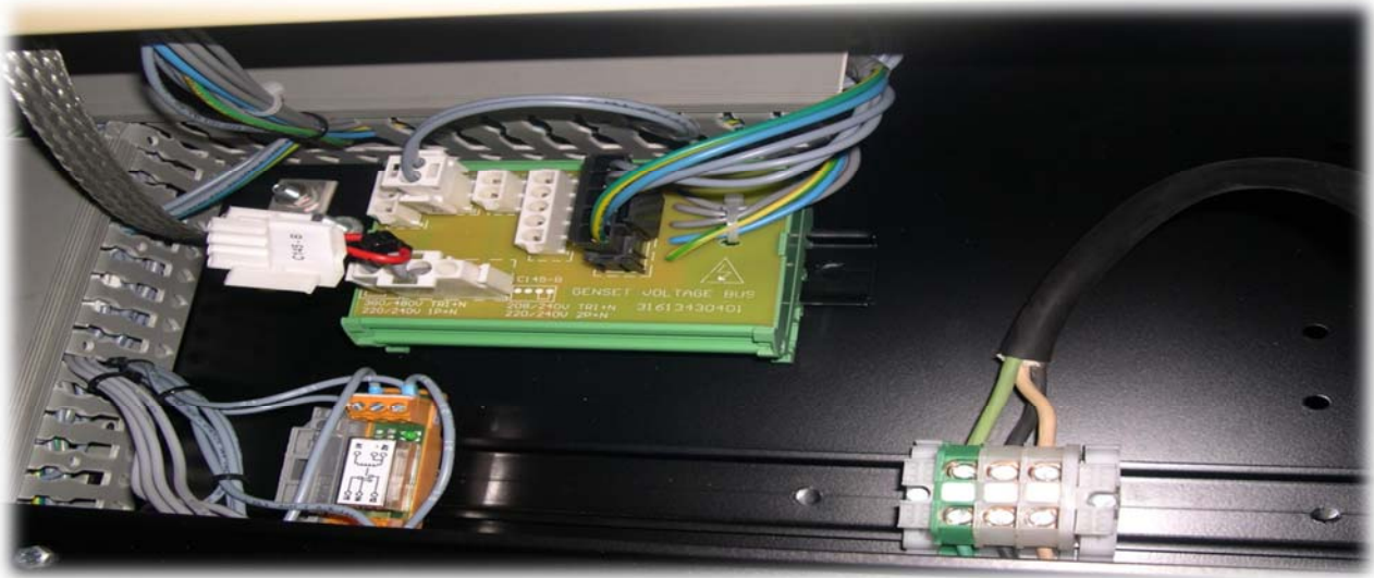
Voltage Bus Distributor Board
