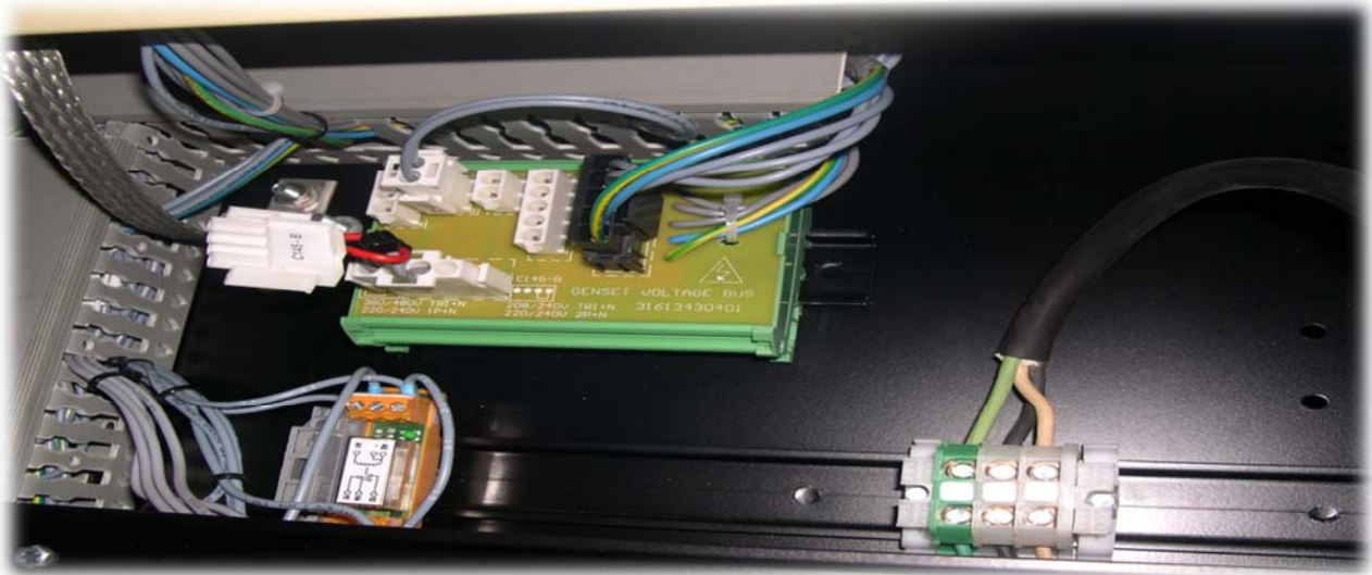
Voltage Bus Distributor Board
