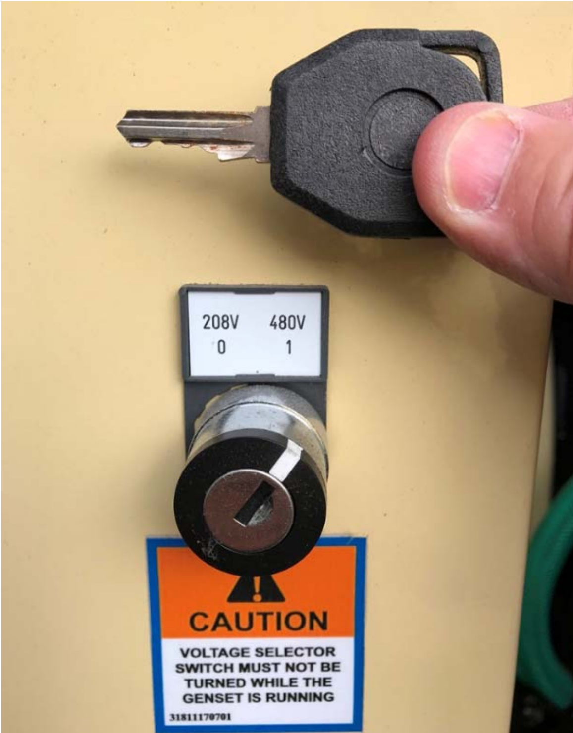
Current Sensing Selector Switch in the 480 VAC position
