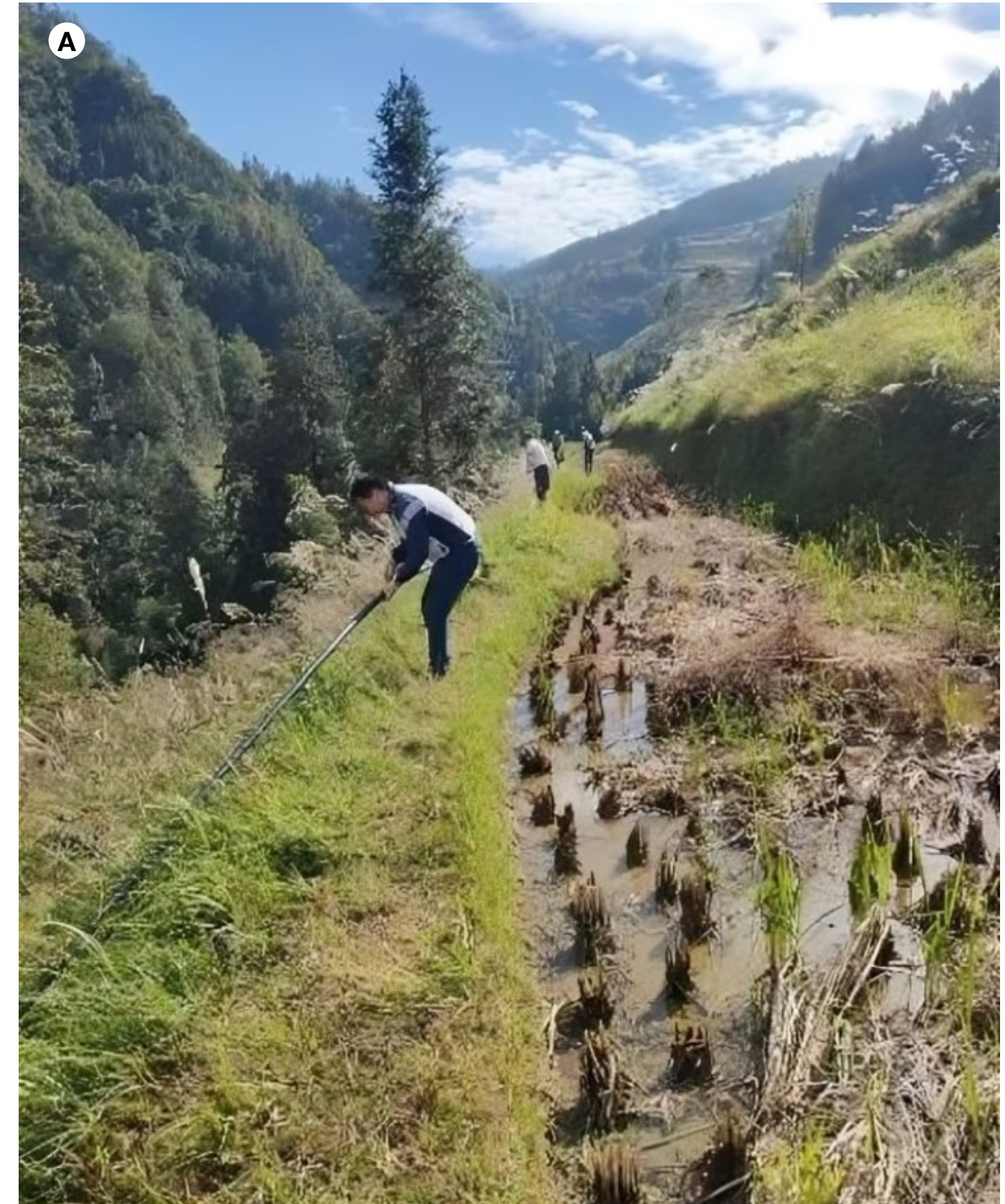
Working to replace pipes and drainage ditches to support clean water access in the Guangxi Zhuang Autonomous Region, China.
