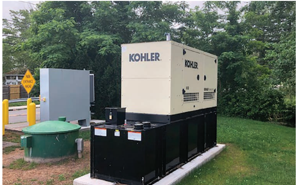
The KOHLER 80REOZJF at a municipal pumping station in East Hampton, Conn.
