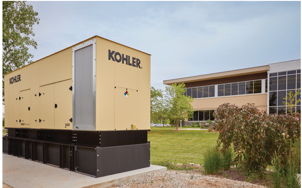
The Kohler 600REOZVB at the Johnsonville Headquarters in Sheboygan Falls, WI
